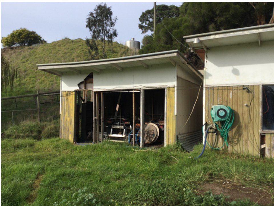
Fig. 14 – View of the existing detached building (previously used as bathroom and toilet) adjacent to the former ski shack
