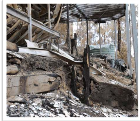
Figure 30 Remains of a retaining wall near a house
